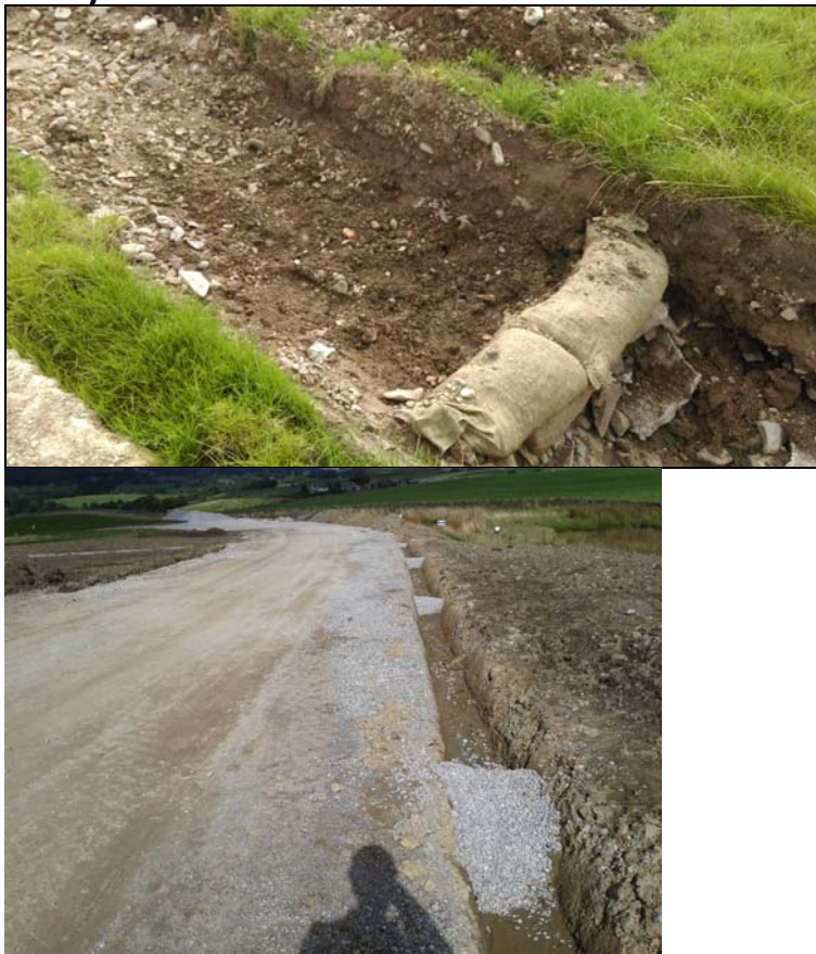
Plate 4: Typical check dams - to be installed in drainage ditches adjacent to the new spine road
