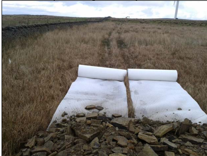
Plate 13: semi-permeable geotextile layer
